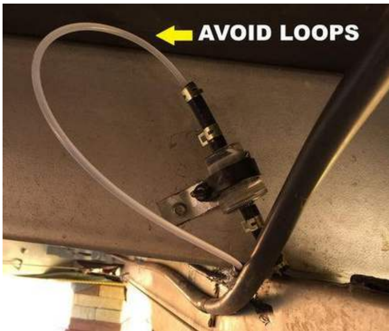
Photo: Improperly routed fuel line
