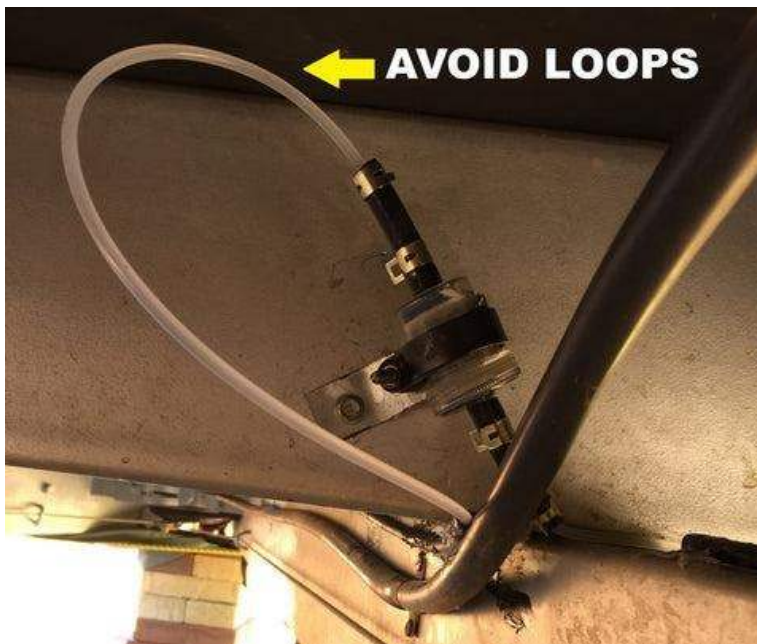
Photo: Improperly routed fuel line
